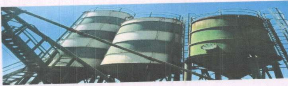
Fig 1. READY MIX CONCRETE PLANT
